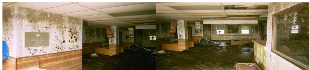
St. Bernard Parish Health Department following Hurricane Katrina, New Orleans, LA. Photograph taken by Daniel Dohony, MPH, CDC Public Health Advisor.
